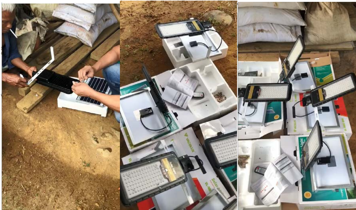
Figure 3.1 The process of transporting PJU poles to the village using a 4 x 4 vehicle due to the rugged terrain (left); The process of installing PJU light poles with residents (right)
