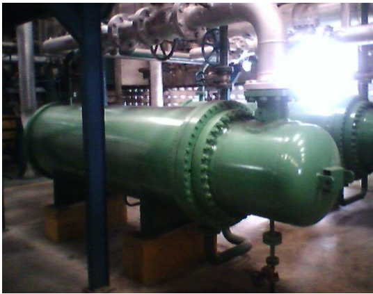
Gambar 1 heat exchanger after cooler
