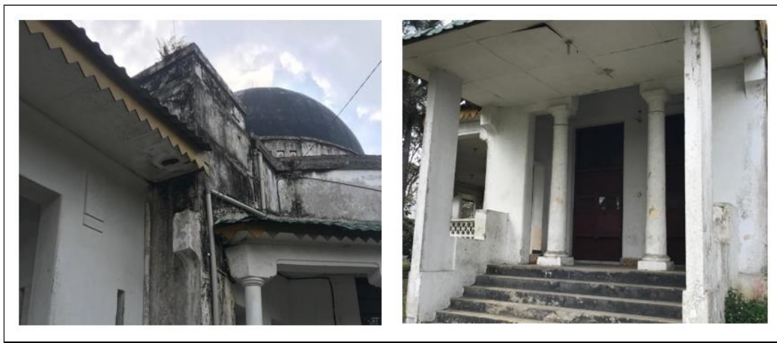
Figure 1. The condition of the Langkat Regional Museum Building
