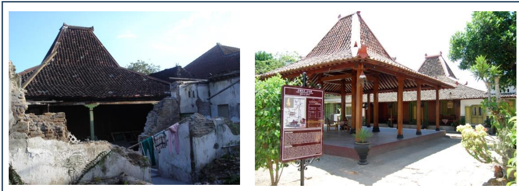
Figure 5 (a) Omah UGM damaged caused by 2006 earthquake (b) Omah UGM recently
