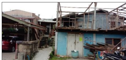
Figure 13 The demolished settlements in Atas Paloh Village
