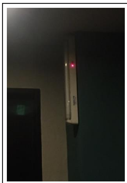
Figure 11. Location of Emergency Lamp
