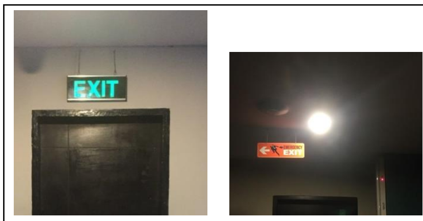
Figure 10. Exit Sign and its Location
