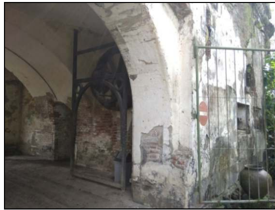
Figure 3. A lift bridge that is no longer visible and only separates the pulley to pull the bridge
