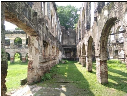
Figure 1. The roof of the fort that was lost and the floor covered by grass
