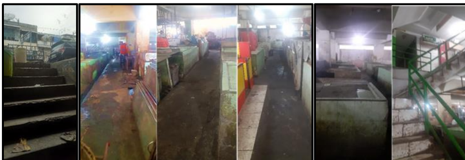
Figure 2 The condition of the basement of the Sukaramai Medan Traditional Market
