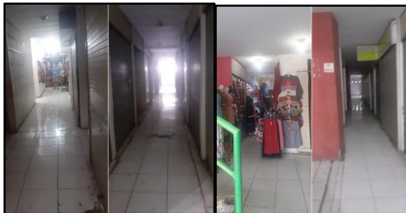
Figure 6 The condition of the second floor of the Sukaramai Medan Traditional Market
