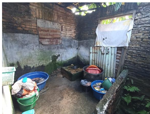
Figure 7. Condition of Semi-Permanent Toilet
