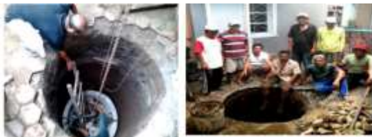
Figure 16. Gotong Royong Residents in Kampung Glintung to Make Infiltration Wells. Source: NUSP2, 2020.
